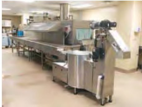
The close coupled pulper and extractor at LeBonheur Germantown Hospital are connected to a soiled tray breakdown station.
